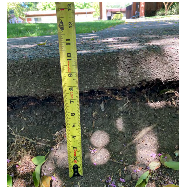
Displaced curb and sidewalk on westbound Berry Street.
