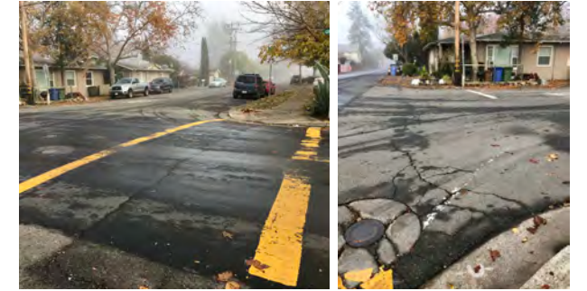
Existing crosswalks (left) are low visibility, while half of the intersection is missing crosswalks (right).
