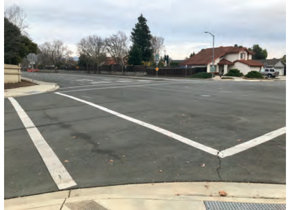
The Chaucer Lane and West American Canyon Road intersection has long crossing distances across American Canyon Road and low pedestrian visibility.
