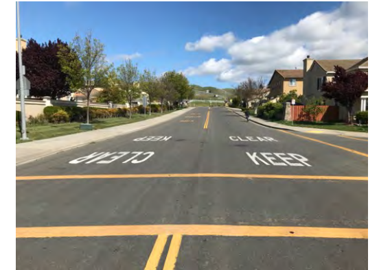
Silver Oak Trail has no bicycle facilities along the entire corridor.
