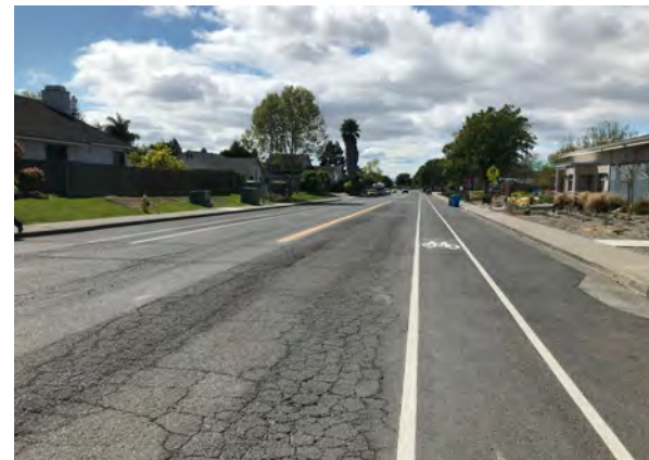
The Class II bike lanes on Benton Way are adjacent to high vehicle speeds and volumes and are frequently crossed by cars pulling up to the curb in the school area.
