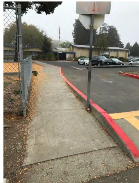
The narrow sidewalk leading to the school's south entrance along its parking lot is narrow and bordered by a fence, forcing pedestrians to step into the parking lot when the sidewalk is too crowded.
