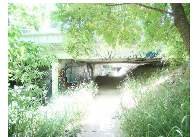
The informal SR 29 undercrossing. Photo credit: Raphael Kluzniok (Napa Valley Register).
