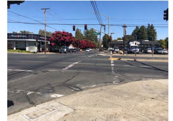
The crosswalks at the Pueblo Ave and Jefferson St intersection are extremely faded.
