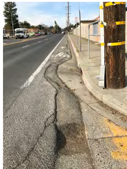
The existing Class II bike lanes on Lincoln Avenue are high-stress, which is exacerbated in areas where the bike lane is narrowed and obstructed by storm drains.
