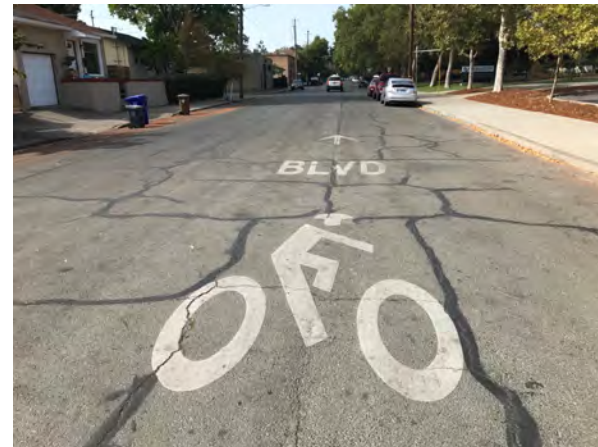
The large sharrows on Yount Street help increase awareness to road users to share the road; however, sharrows alone do not reduce the stress of high traffic volumes/speeds in the school zone, particularly during peak school hours.
