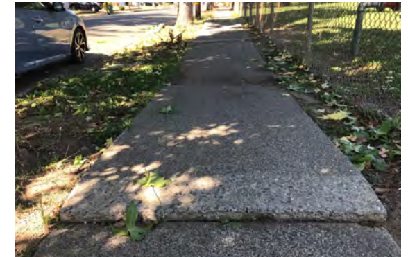
The northbound Linda Vista sidewalk is displaced in multiple locations.
