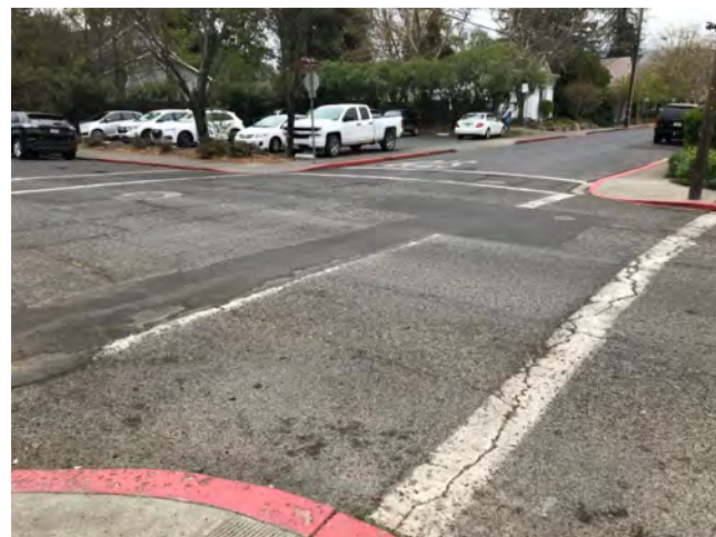
Poor road quality at Oak Avenue and Pine Street discourages bicycling.
