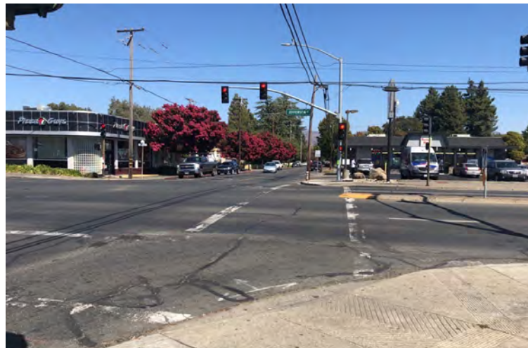
The crosswalks at the Pueblo Ave and Jefferson St intersection are extremely faded.
