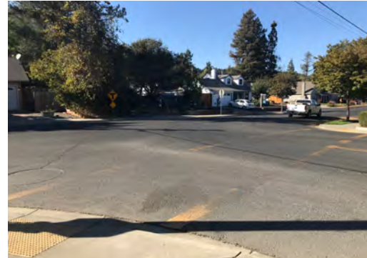
The crosswalks at Foster and Imola are extremely faded.
