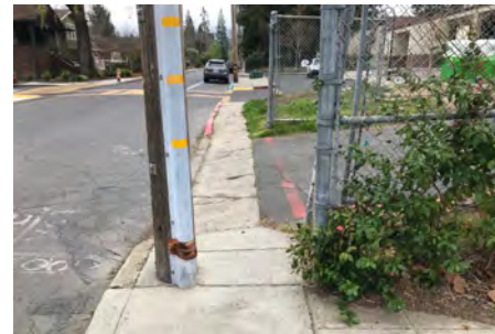
Narrow sidewalks on Tainter Street are not ADA-accessible.
