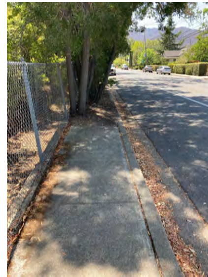
One of the locations where the sidewalk ends on eastbound Spring Street with no crosswalks to the existing westbound sidewalk.
