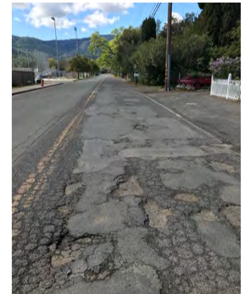
Poor road quality on Grayson Avenue.
