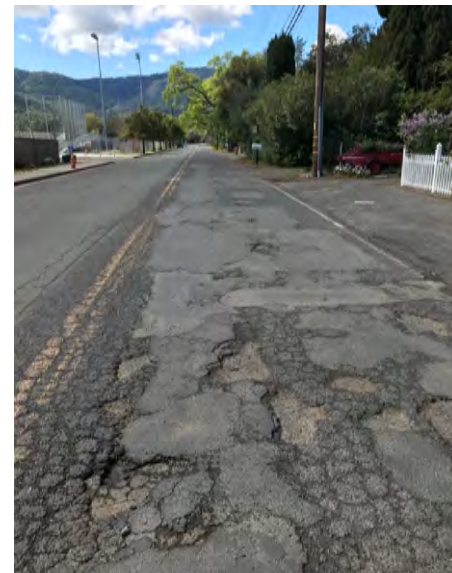
Poor road quality on Grayson Avenue.
