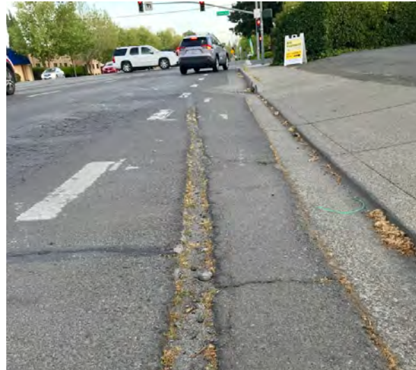
The divot in the southbound bike lane is a fall hazard for bicyclists.
