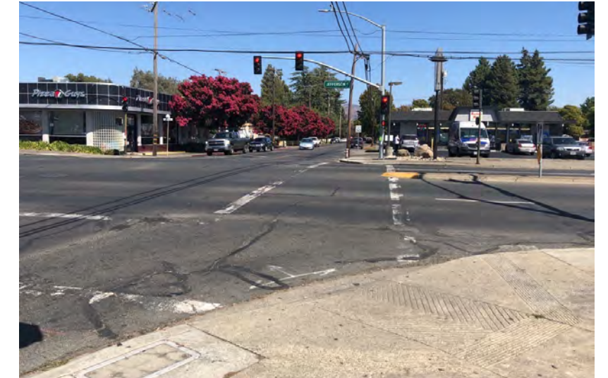
The crosswalks at the Pueblo Ave and Jefferson St intersection are extremely faded.
