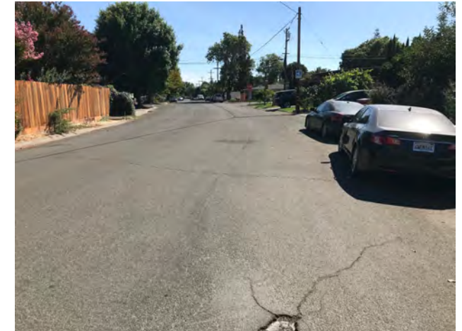
Carol Drive has no sidewalks or bicycle facilities.
