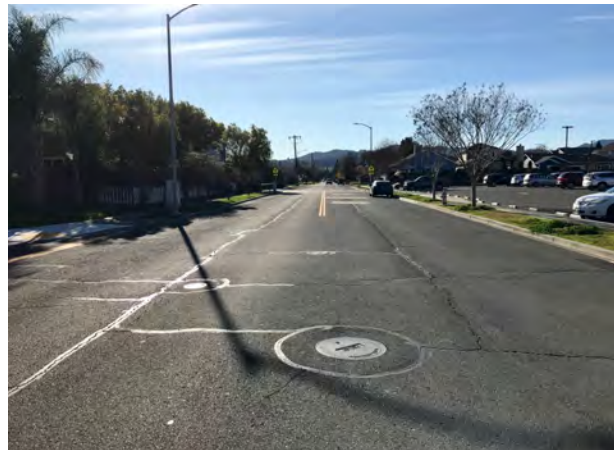
There are no bicycle facilities on El Centro Avenue.
